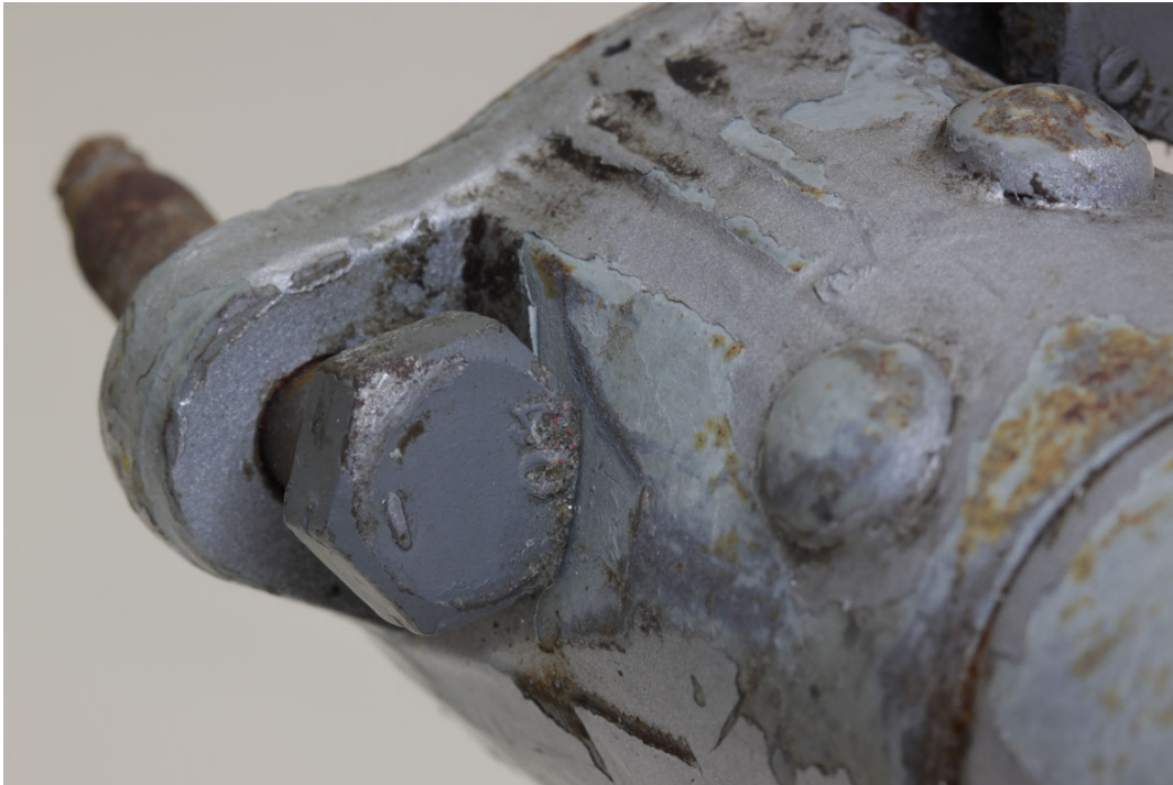
Figure A9: Bolt on right side showing head markings
